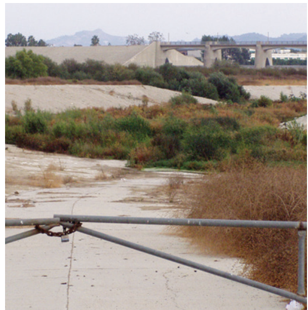
Improvement of flood control channels is being considered to achieve IRWMP objectives.
